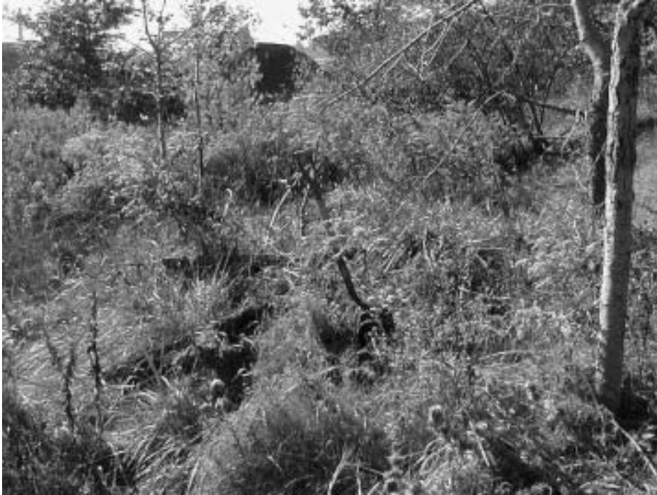
Figure 2. A mound of sand covering a stormwater discharge pipe from Interstate I-190. The mound is covered with grass and weeds. Note size of shovel for scale.
