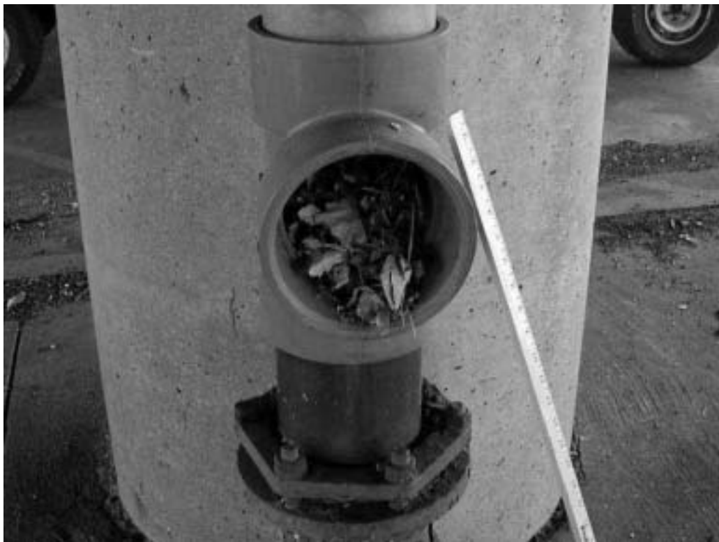
Figure 1. Example of poorly maintained stormpipe from Interstate I-190 overpass. Note pipe is completely clogged with sediment and debris.
